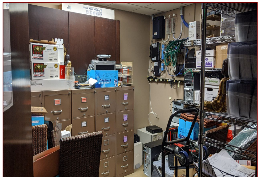
Storage / Server Room
